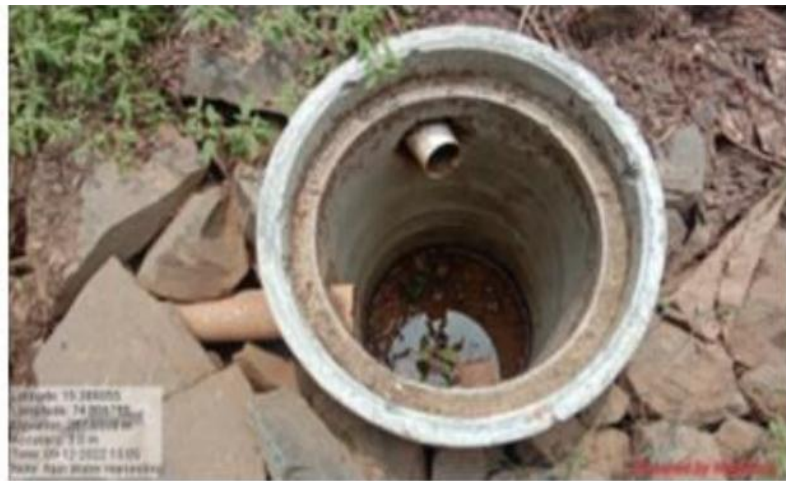
Ground Water recharge unit installed at the behind principal's office
