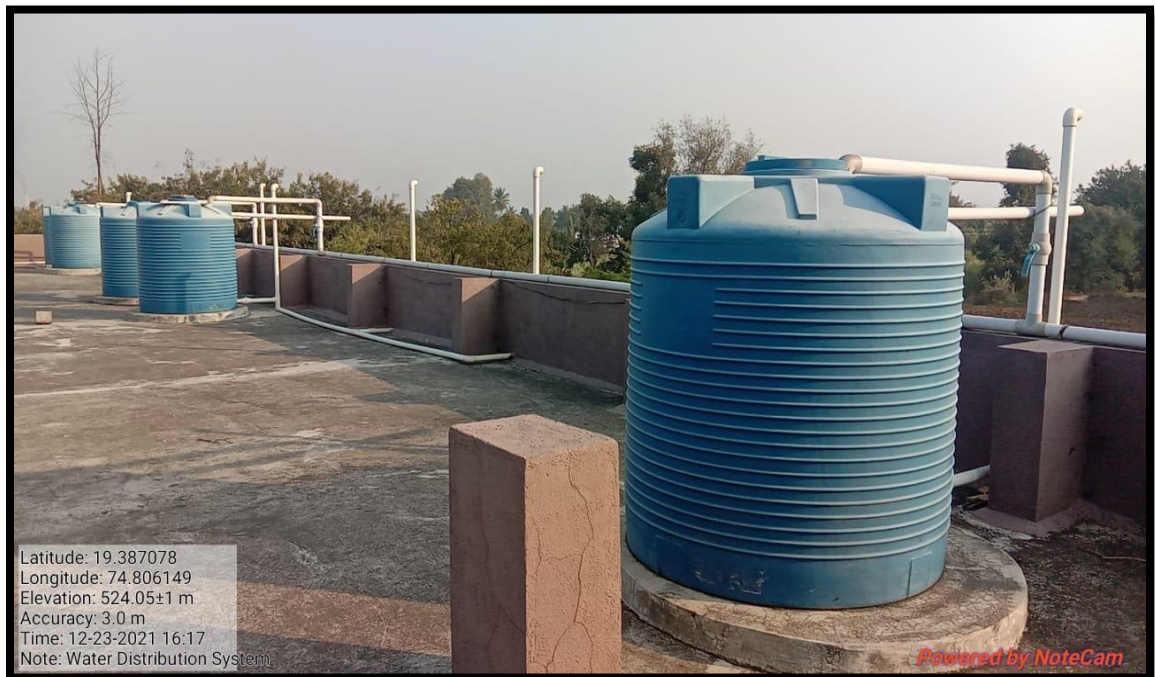
Water Distribution System in College Campus.
