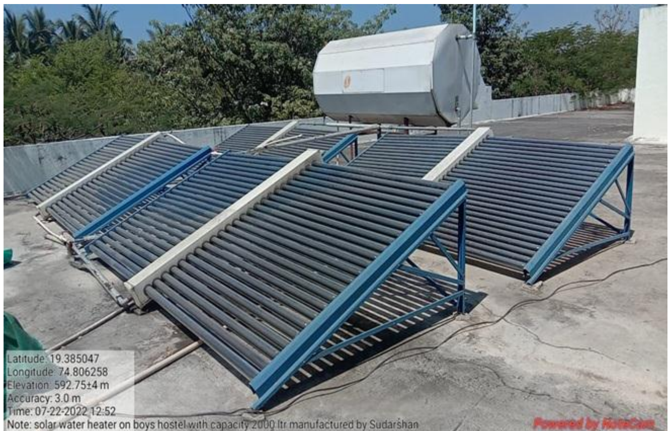
Solar Water Heater on Boys Hostel (Capacity: 2000 Ltr)
