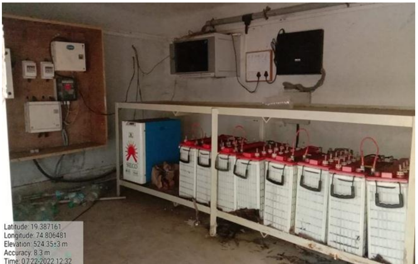
Inverter System of Solar Panels in Vidnyan Bhawan
