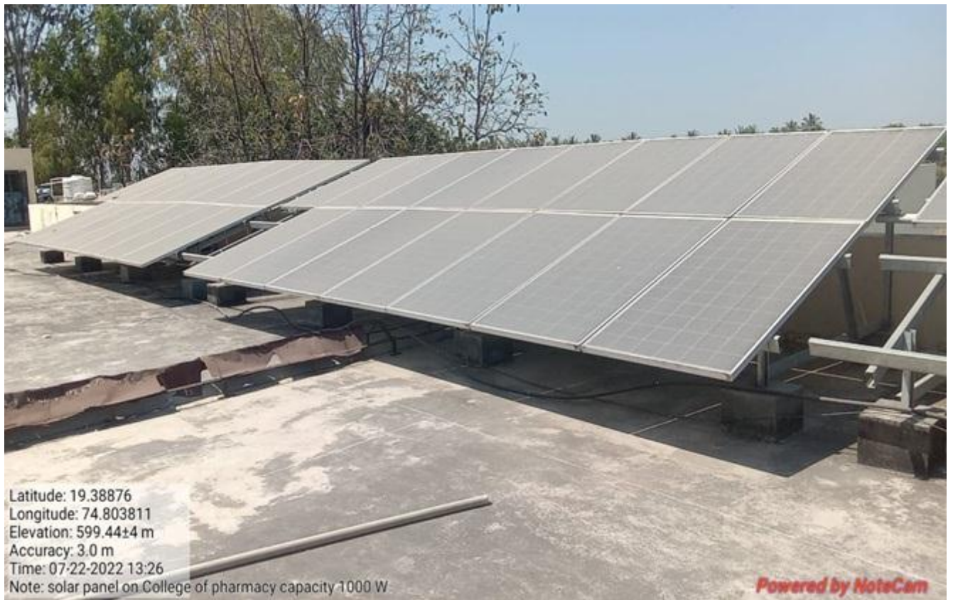
Solar Panels in Mula Education Society's Campus (Capacity: 10 KW)
