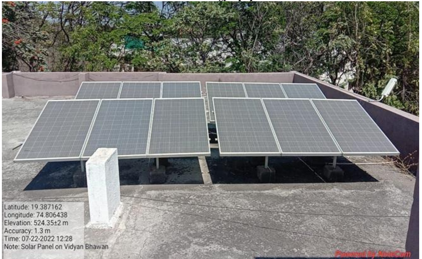
Solar Panels on Vidnyan Bhawan (Capacity: 1 KW)
