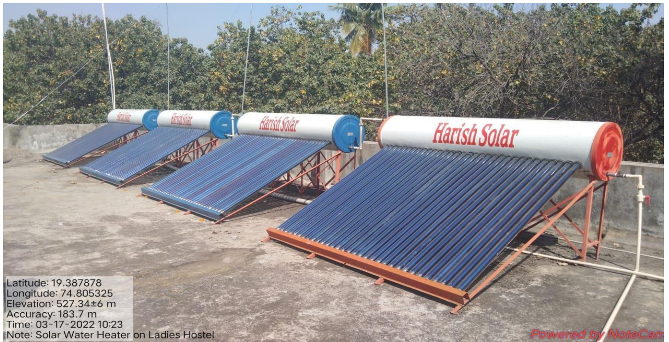
Solar Water Heater on Ladies Hostel (Capacity: 4000 Ltr)
