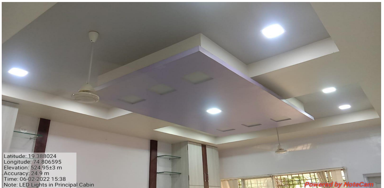
LED Lights in Principal Cabin
