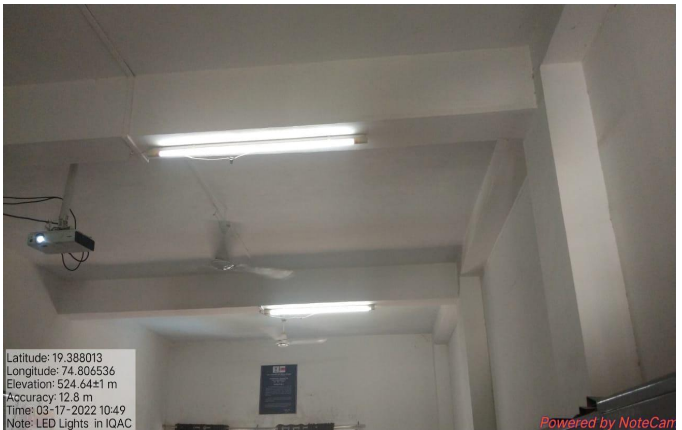
LED Lights in IQAC
