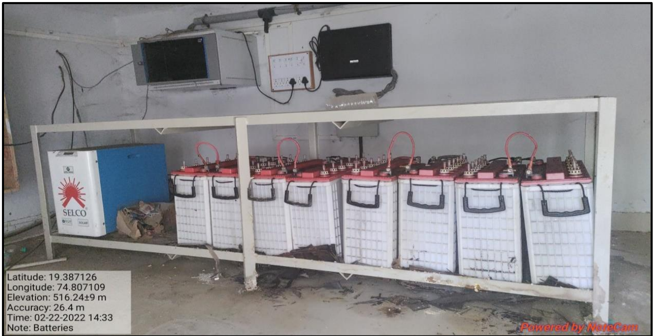
Batterie and Inverter for Solar PV system (1 KW)
